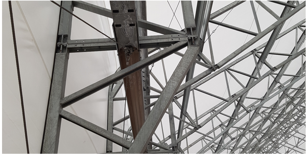
Source: Calhoun Super Structure, 2018
