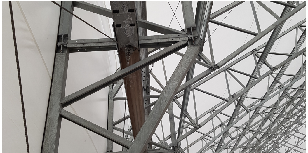
Source: Calhoun Super Structure, 2018
